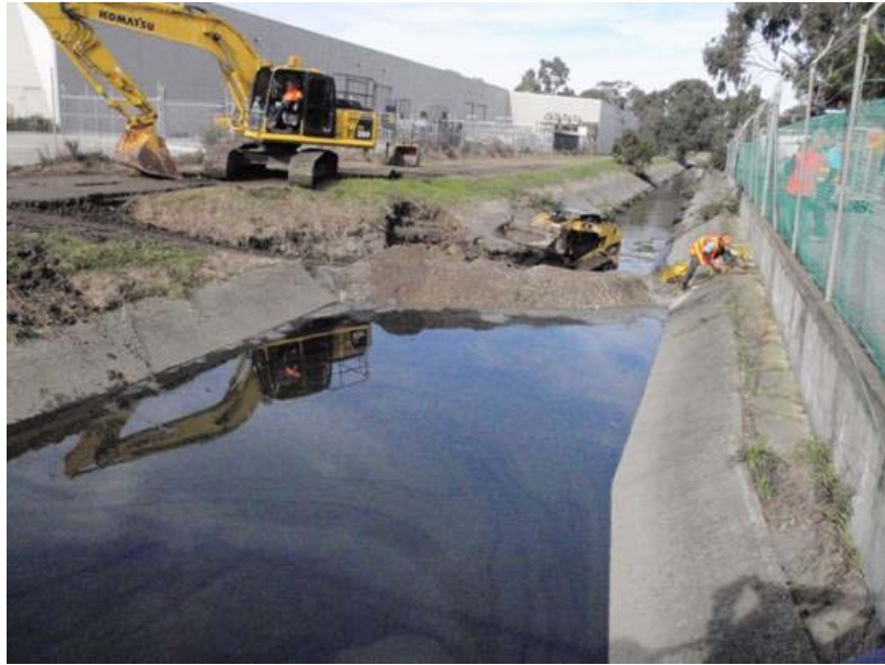
Figure 7. Sand bunding used to contain oil and contaminated water run-off (Source: Melbourne Water)
