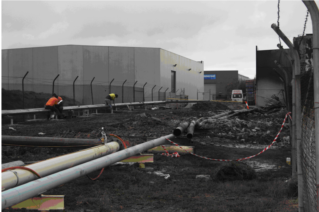
Figure 3. Hydrogen, nitrogen and compressed air pipelines located to the rear of TriTech (K Pakenham, CFA)
